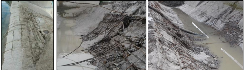
Fig. 2 Damaged reinforcement of the weir's glacis (a) and of the stilling basin (b and c).
