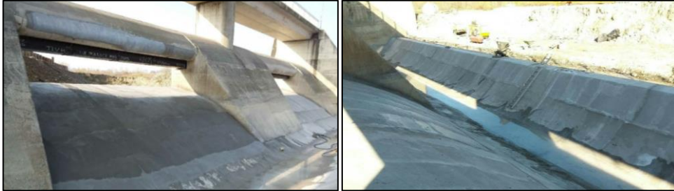
Fig. 3 Weir's glacis (a) and stilling basin (b) after the intervention.
