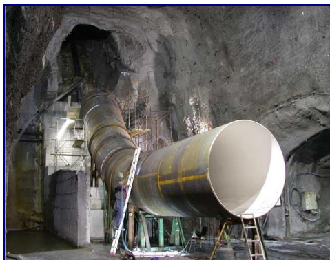
Premadio II HPP – Penstock (Alps)
